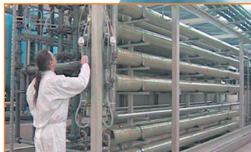
Reverse-osmosis 3.000 m 3 /day
