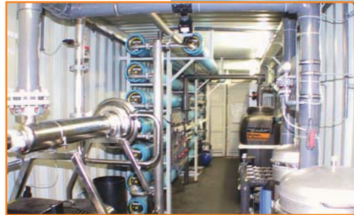
Seawater desalination 500 m 3 /day
