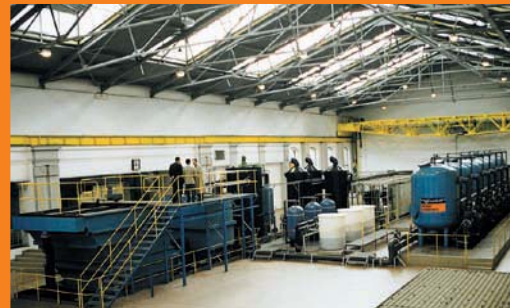
Water works 5.000 m 3 /day
