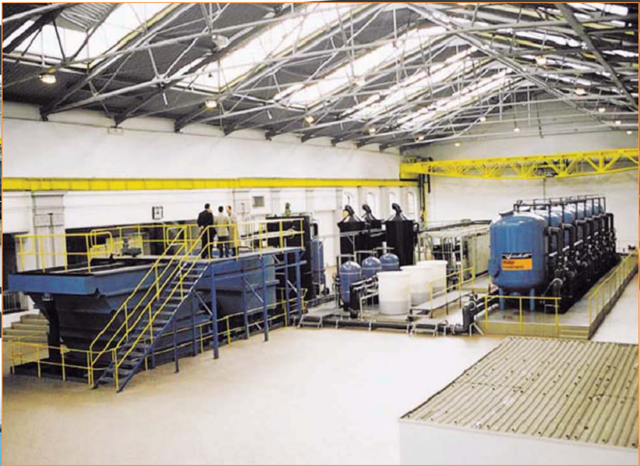
Customized plant in overview
