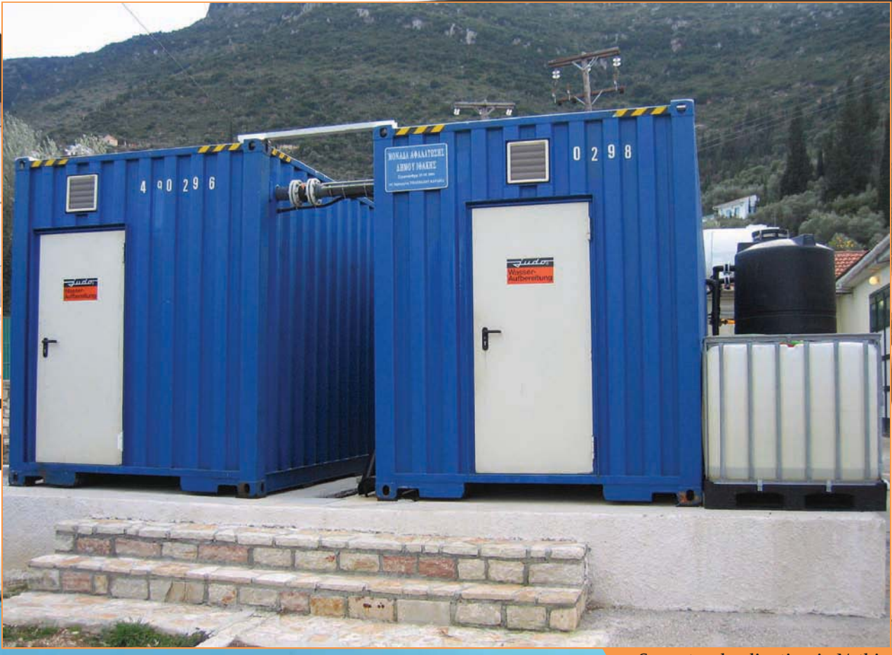
Seawater desalination in Vathi
